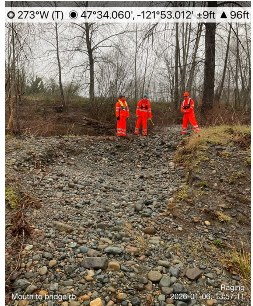
King County staff inspecting damage along the Raging River, Jan. 6, 2026
