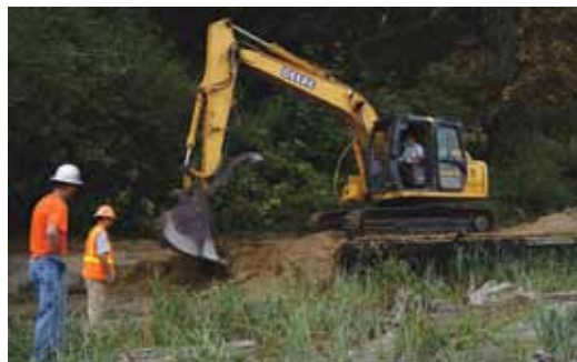
A decaying, creosote-soaked bulkhead on Piner Point on Maury Island was removed in the summer of 2010. Removal will allow the bluff to erode naturally to feed sediment to the beach.
