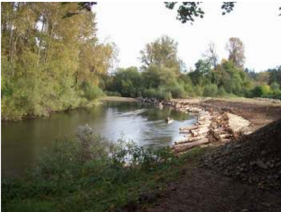
Restoration work in progress just upstream of the proposed phase of work.
