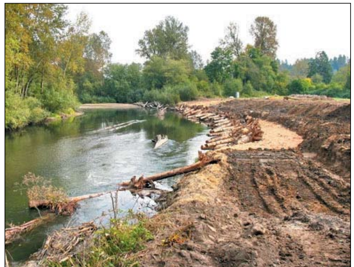
The Fenster restoration in Auburn under construction in October 2008, showing large wood used to armor the toe of the bank while providing shelter for fish. Photo courtesy of King County.
