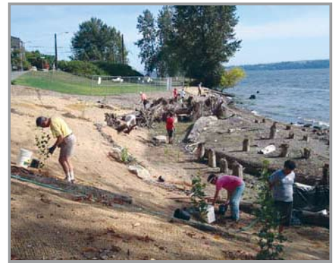
Friends of Madrona Woods transformed Madrona Park Creek from an underground pipe into almost 1,400 feet of open stream channel, installed a fish passage culvert, and created 400 feet of shoreline cove along Lake Washington.
